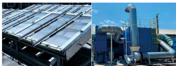
Fig.1 Deodorization and degreasing system.
