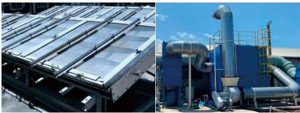
Fig.1 Deodorization and degreasing system.
