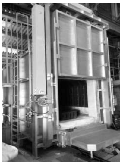
Fig.8 Heat treating furnace
