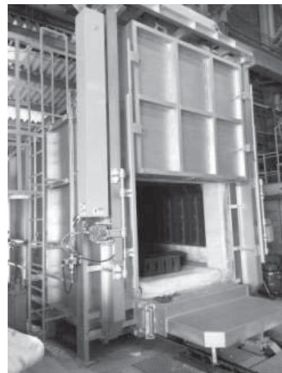
Fig.8 Heat treating furnace
